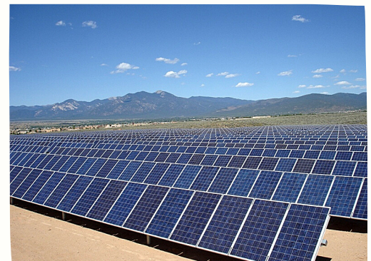
University of New Mexico Klauer Campus, 500kW PV array
